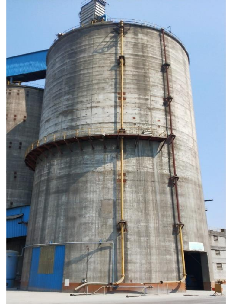
Multi Compartment Silo
